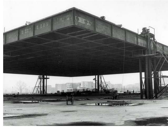
1967. Mies van der Rohe, Neue Nationalgalerie. The steel roof structure for the Neue Nationalgalerie was raised by hydraulic jacks and then lowered onto eight supports. © SMB, Zentralarchiv
