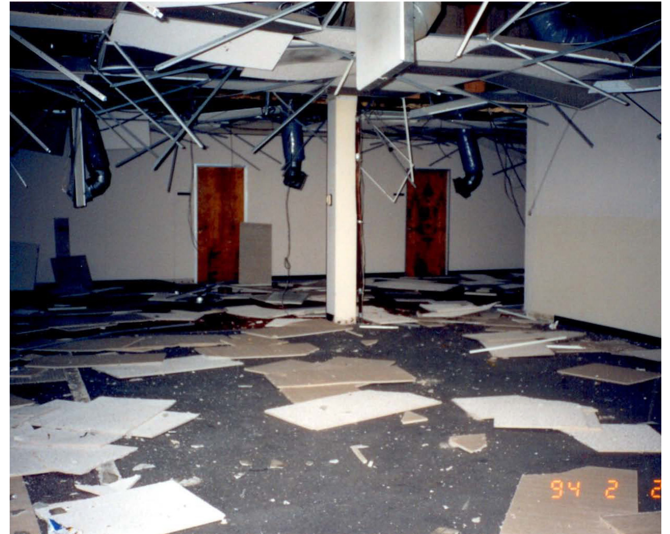
1994. "Dropped" Ceiling. Failure of suspended ceiling system including lights and air diffusers in the Northridge Earthquake (Photo credit: Wiss, Janney, Elstner Associates). US FEMA Earthquake planning, Chapter 6.3.4.1 "Suspended Acoustic Lay-In Tile Ceiling Systems. January 2011.
