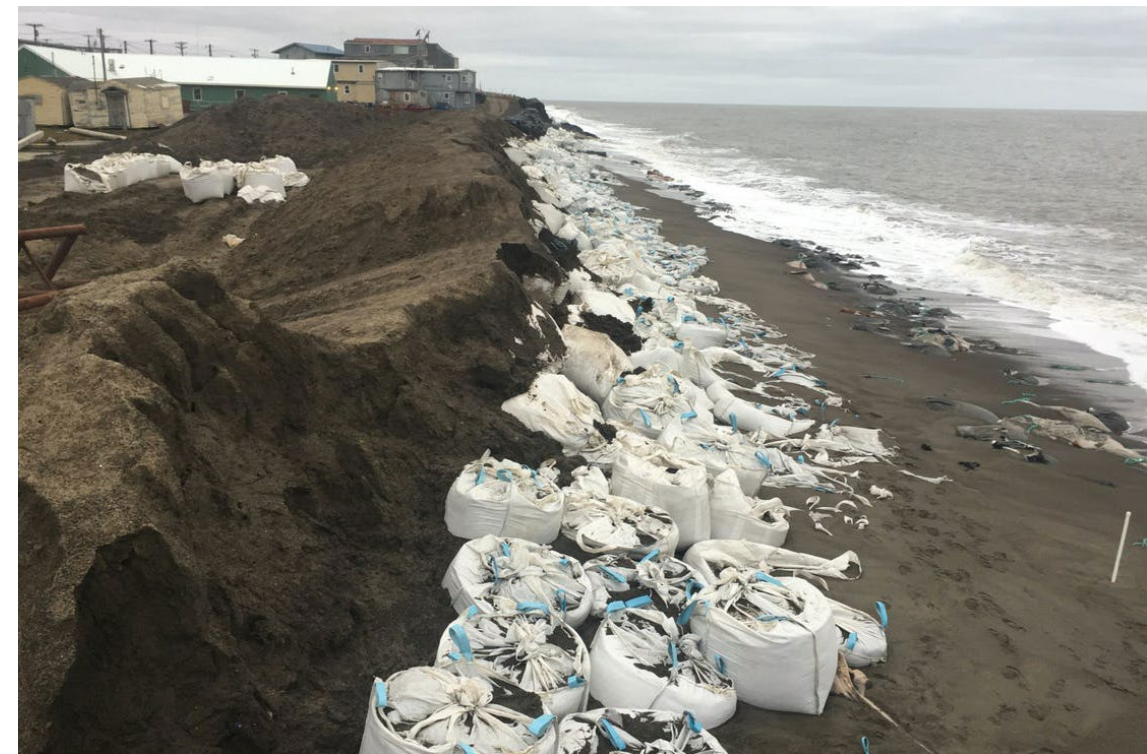
FIG. 46 Coastal erosion Utqiagvik, Alaska.
