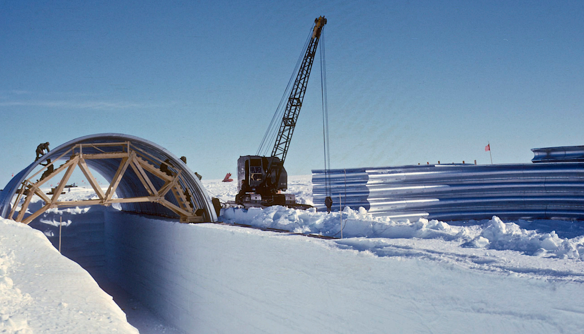
Newly cut trenches in the Greenlandic ice sheet are being covered with corrugated steel arches, Camp Century, 1962.
