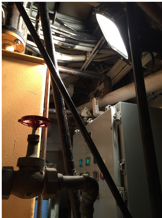
Figure 24. 500W halogen light in Forward Engine Room (FER). Figure shows light directed away from crew traffic and task areas to avoid glare and heat when working nearby. Several 500W lights were positioned away from task areas, providing light where services were not required.
