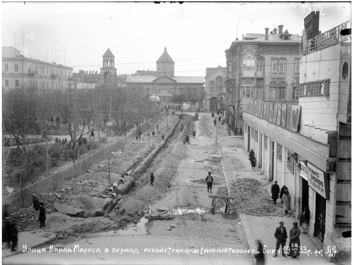
FIGURE 3.13: Karl Marx Street (пр. Зии Буньятова) during reconstruction, February 20, 1933 Photo: L. Bregadze Azerbaijan State Kino-Foto-Fono Archive, Inv. 5-243
