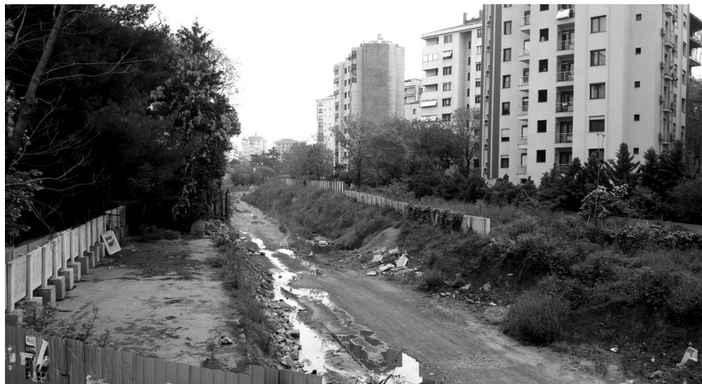
Figure 4.13: The current condition of the Marmaray Railway. The construction has been delayed due to disputes related to the tender.
