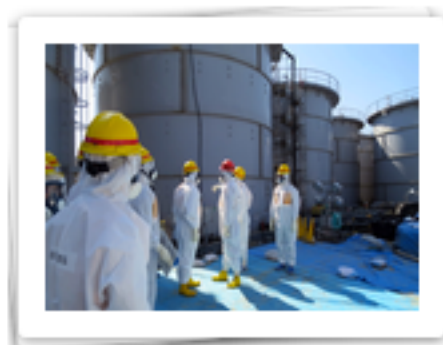
Radioactive water leakage (2013)
