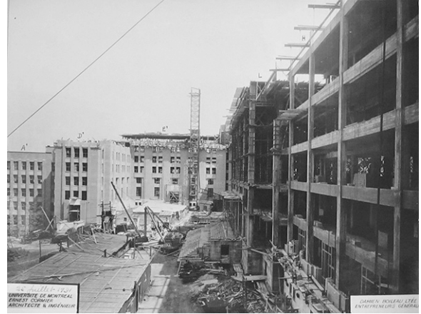
Figure 6.33 A photograph of the central zone of the main pavilion under construction, dated July 25, 1931. Source: S. J. Hayward, P.1846, “Pose de la brique ailes D’ et E’. Perrons d’honneur aile L, étages 4, 6, 9 aile L étages 3 à 9 aile H,” box 02-2402-01P, FEC, CCA.
