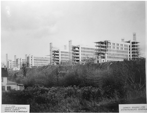
Figure 5.11 A photograph of the front wings of the main pavilion under construction, dated November 8, 1930. Source: S. J. Hayward, “Vue des façades C', B', A', A, I, B, J, C et vue du solarium sud de D,” P.1848, box 01-2402-01P, FEC, CCA.
