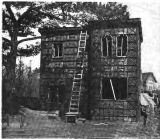
FIG. 5—THE FORMS ALL IN PLACE READY FOR POURING. Note the runway to the mixer platform at the right of the building.
