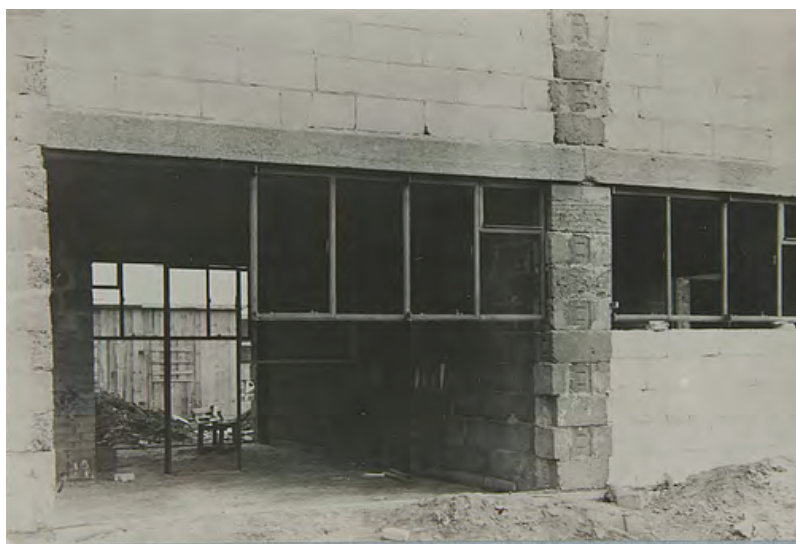
Fig. 162. Photographs showing cracking in Type II facades, due to the use of large format pumice panels, which had not adequately cured, before being installed, in 1928 (top) and photographs of experimental Type IV units with smaller pumice panels in 1929 (middle, bottom). Source: "Bericht Über Die Versuchssiedlung in Dessau." RFG Sonderheft Nr. 7, no. Gruppe IV NR. 4 (April 1929).
