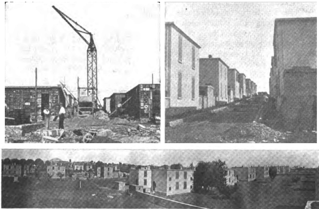
Fig. 66. Plates from Harms, "Building Concrete Industrial Houses by Harms System in France", showing two progress photos, taken one week apart, of pouring sequence along one of the street at Salindres (top) and view of the completed street (bottom). Source: Harms. "Building Concrete Industrial Houses by Harms-System: Second Article Describes Layout of Work, Equipment and Methods Used." Concrete 12, no. 2 (February, 1918): 41-46.
