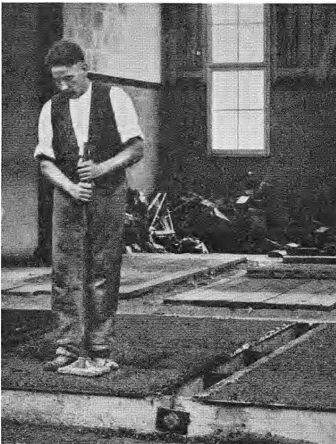
Fig. 191. Plates from Das Neue Frankfurt showing simple, adjustable formwork used in casting Frankfurt system panels (top) and the manual stamping, required by the SPD (bottom).
