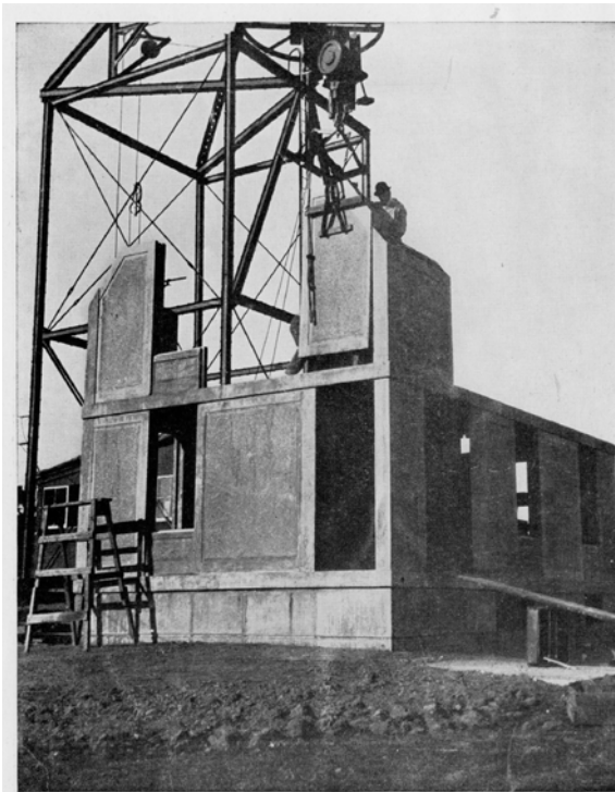
Setting Wall Block, Third Tier. Crew Consists of Hoisting Engineer, Foreman and Two Laborers. House Erected in Fifteen Working Days.
