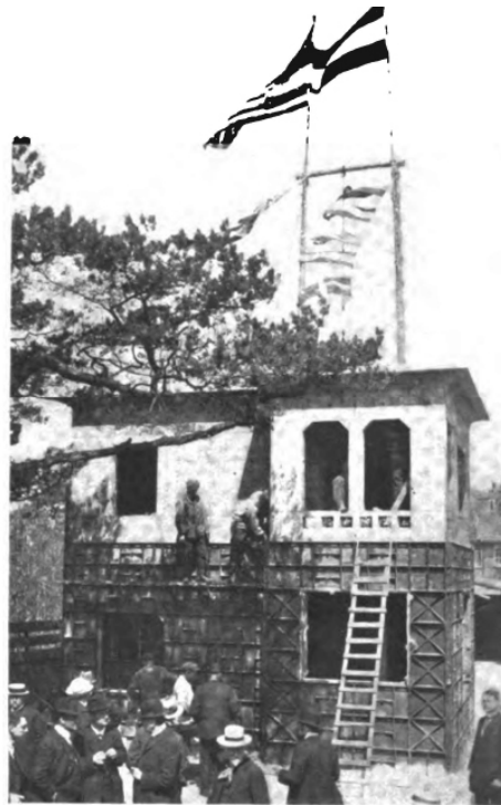
FIG. 7—REMOVING FORMS. The flags are flying from the concrete tower. Indressed timber is used for scaffolding.
