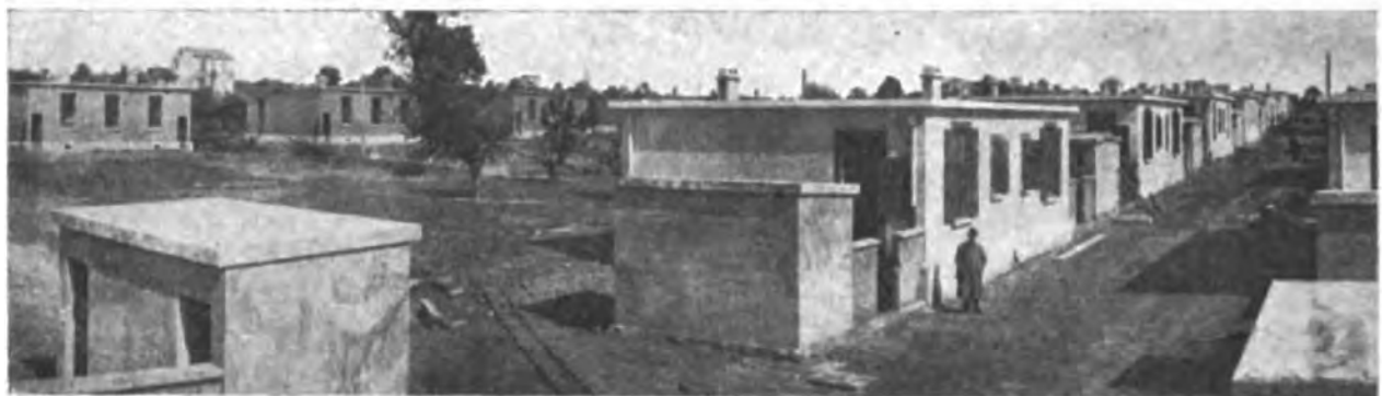
Fig. 67. Plates from Harms, "Building Concrete Industrial Houses by Harms System in France", showing two progress photos, taken one week apart, of the erection of molds, with precast floor beams, in foreground (top and middle) and view of the completed street (bottom).
