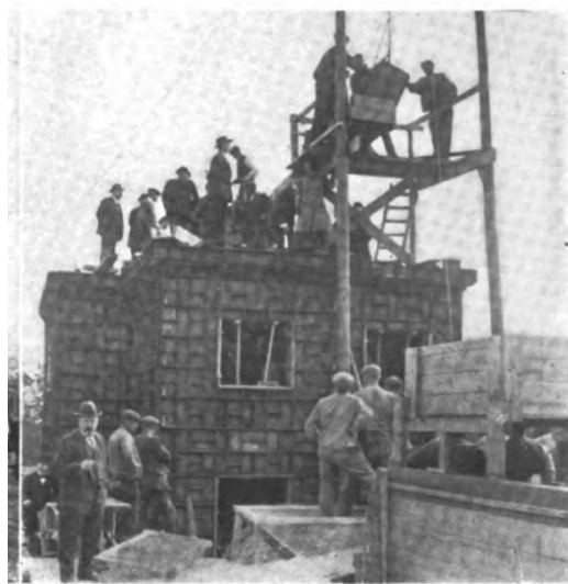
FIG. 6—POURING A MONOLITHIC HOUSE. The concrete, very wet, is hoisted to the platform, and emptied into a tank, from which it pours into the forms.
