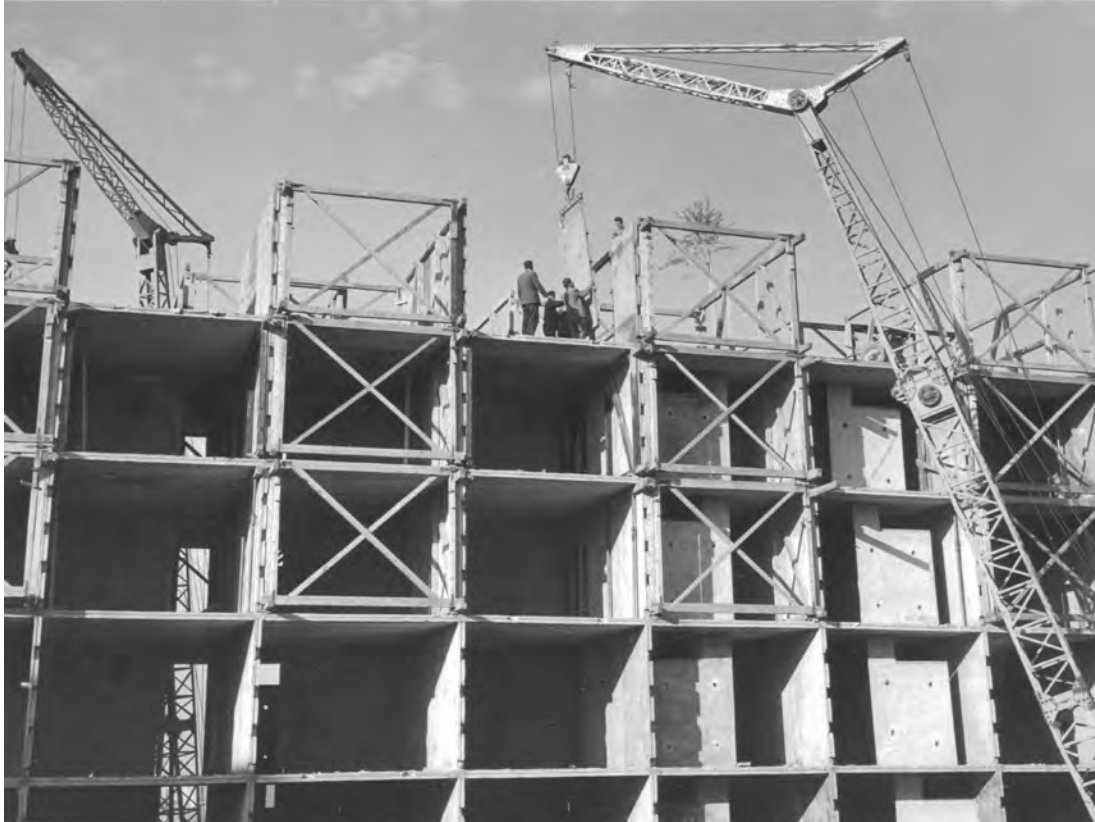
Fig. 235. Assembly of JU 61 System, showing the universal floor and wall panels and a system of reusable wooden centering forms, 1963. Source: Private Archive, Bogdan Budimirov.
