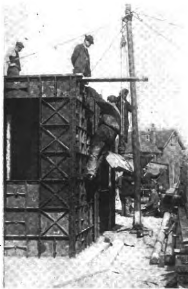
FIG. 4—PLACING A SECTION OF THE PRE-CAST FLOOR. The floor is pre-cast in units and assembled when the forms are placed.
