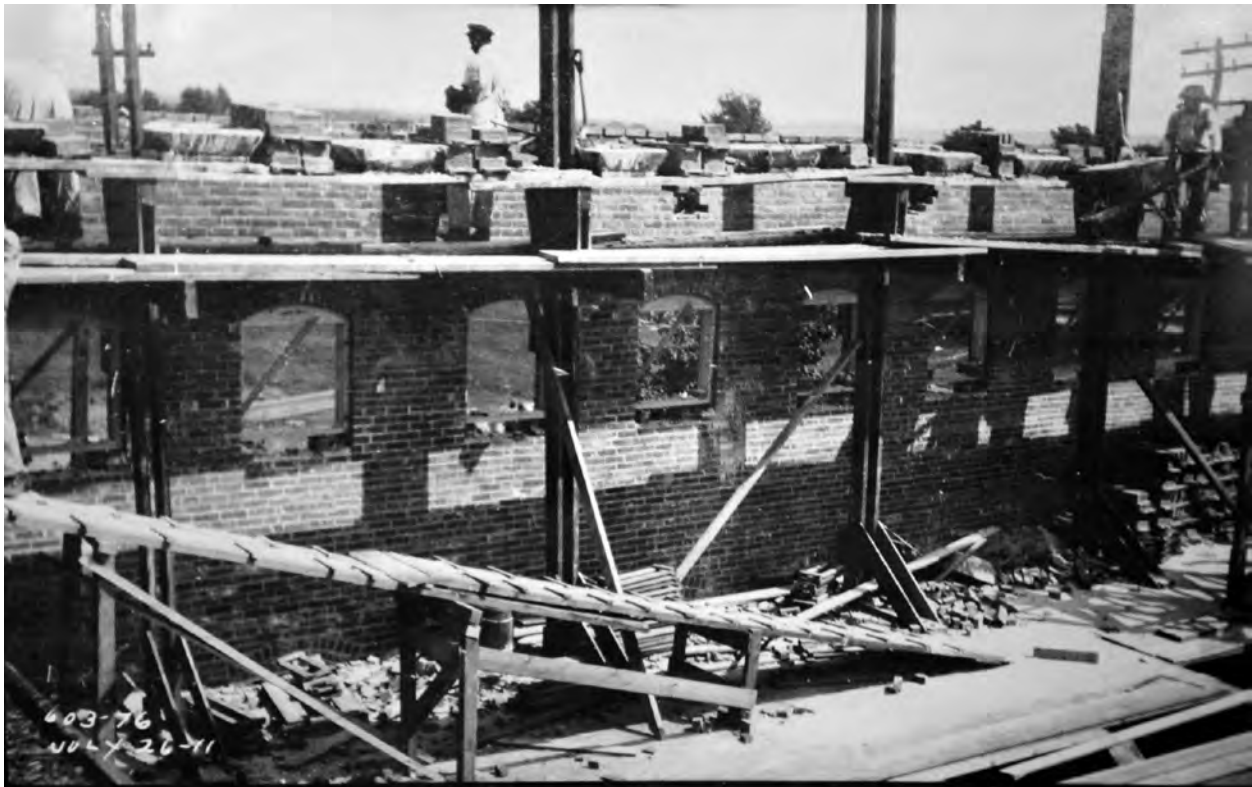
Fig. 19. F. Gilbreth, progress photos of Gilbreth scaffold, installed on a construction site in Boston, MA, July 1911. Source: FLGA Box 146 Photographs, undated Folder 0028 v. II 2 bricklaying and factory studies Photos 603-30, 603-76.
